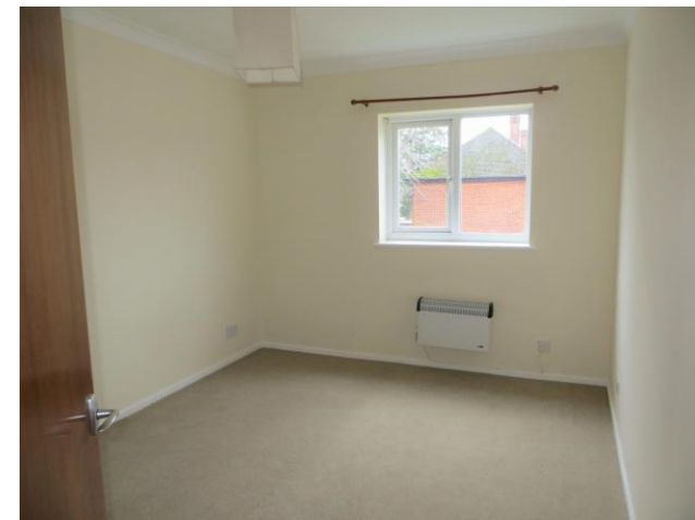
BEDROOM TWO: double glazed window, electric wall heater.
